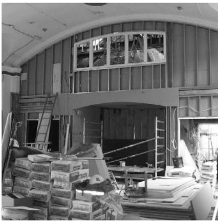
View of the new Bradbury Room from the Hall with its window in place, with the servery, podium and store underneath.
