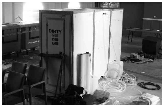
The builders have begun! An Asbestos Removal Unit sits in the Hall. The door on the other side of the unit says 'Clean'!
